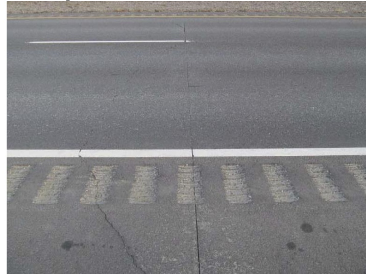
Photo: Pre-cut pavement section on the Richardson Highway near Moose Creek. Photo credit Bob McHattie and Dr. Jenny Liu.
