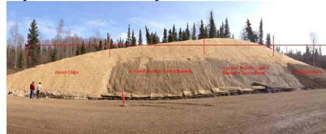
Test sections constructed on the Dalton Highway 9 Mile Hill North project. Photo credit AUTC.
