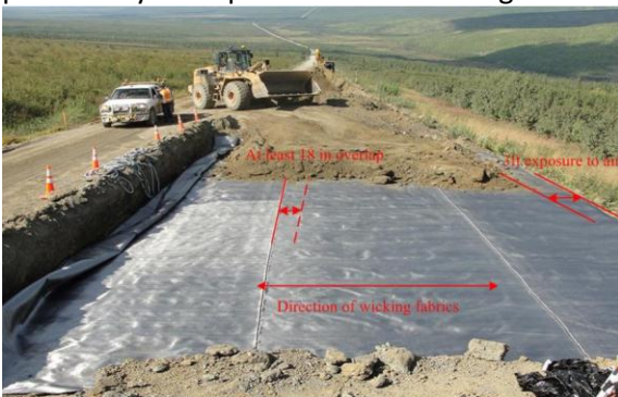
Photo: Wicking fabric installation at Dalton Highway MP 110.5 Beaver Slide. Photo credit AUTC.
