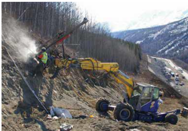
Drilling of the soil and rock slope on Glenn Highway Photo: Terry Barber
